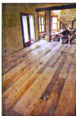
A worker looks over worry chestnut planks installed as the kitchen floor of the Sancic home.
