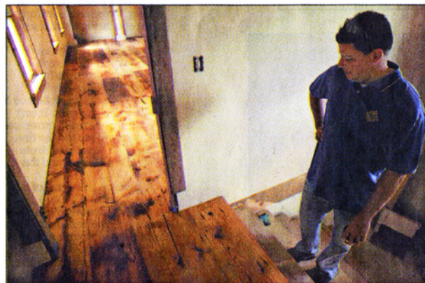
Tommy Sancic looks over pine planks with an especially pronounced grain used in the upstairs hallway and guest room.
